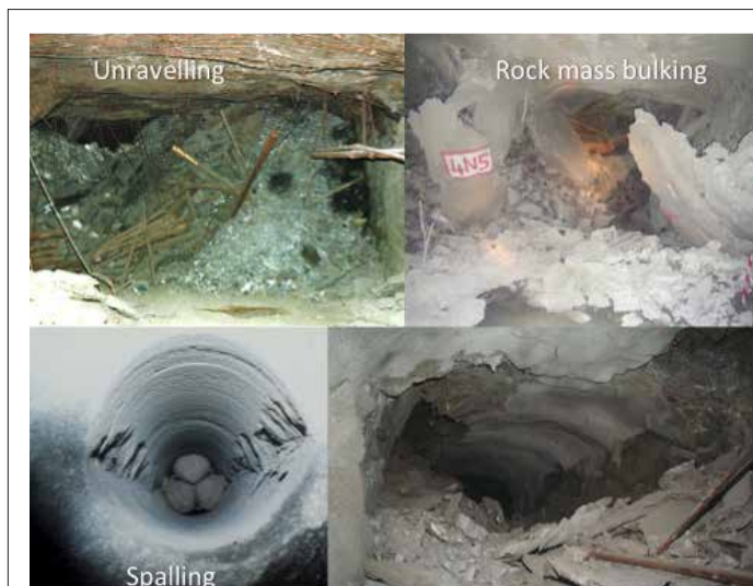
Figure 11: Examples of excavation instabilities in stressed rock
